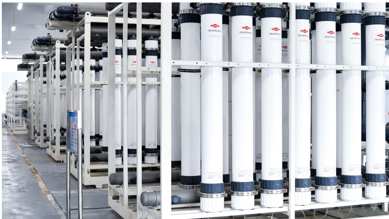
The Wastewater Resource Utilization and Emission Reduction Device (Membrane Treatment) of Yunnan Shuifu Yuntianhua Co., Ltd
