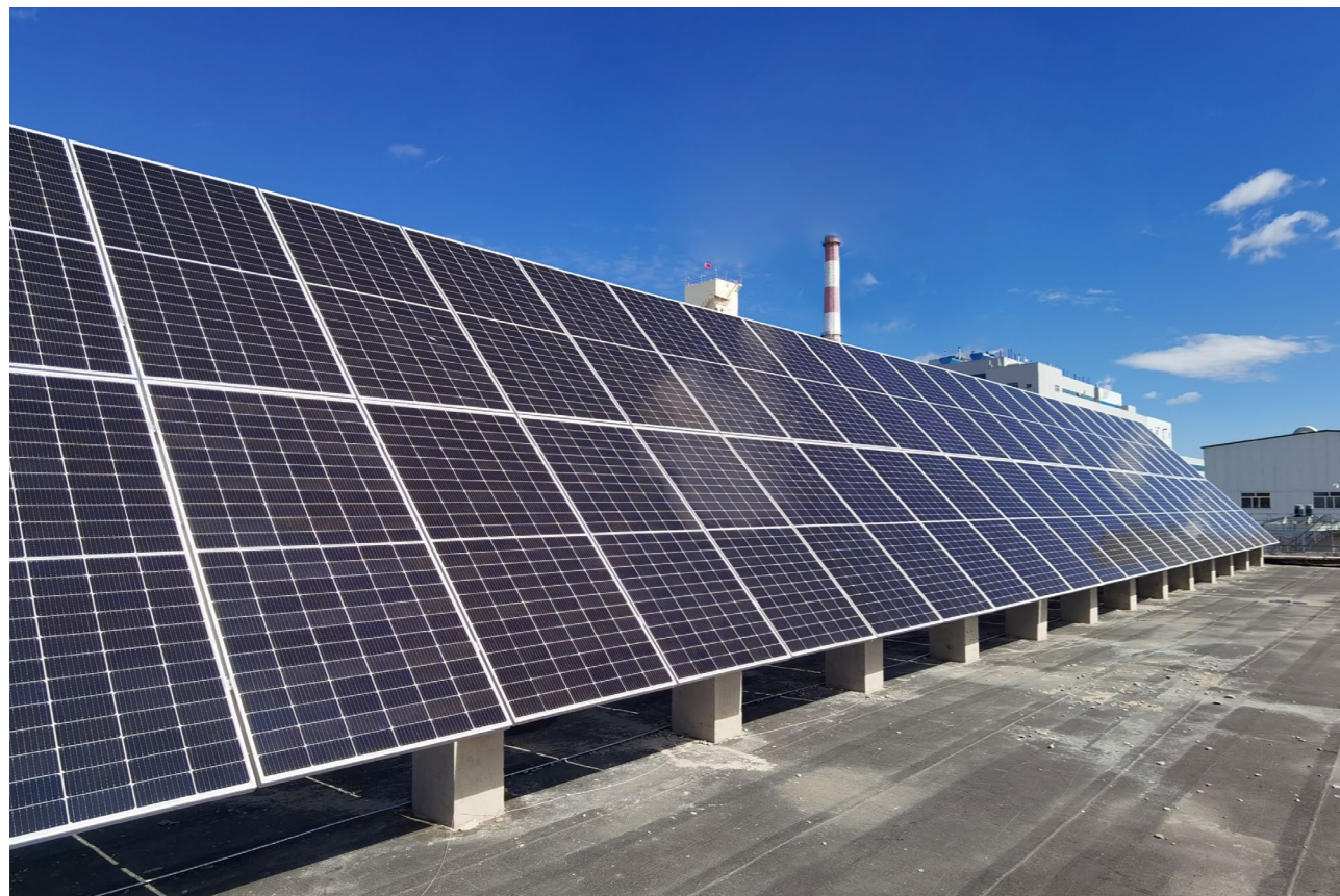
Plant Roof Photovoltaic in Jinxin Chemical
