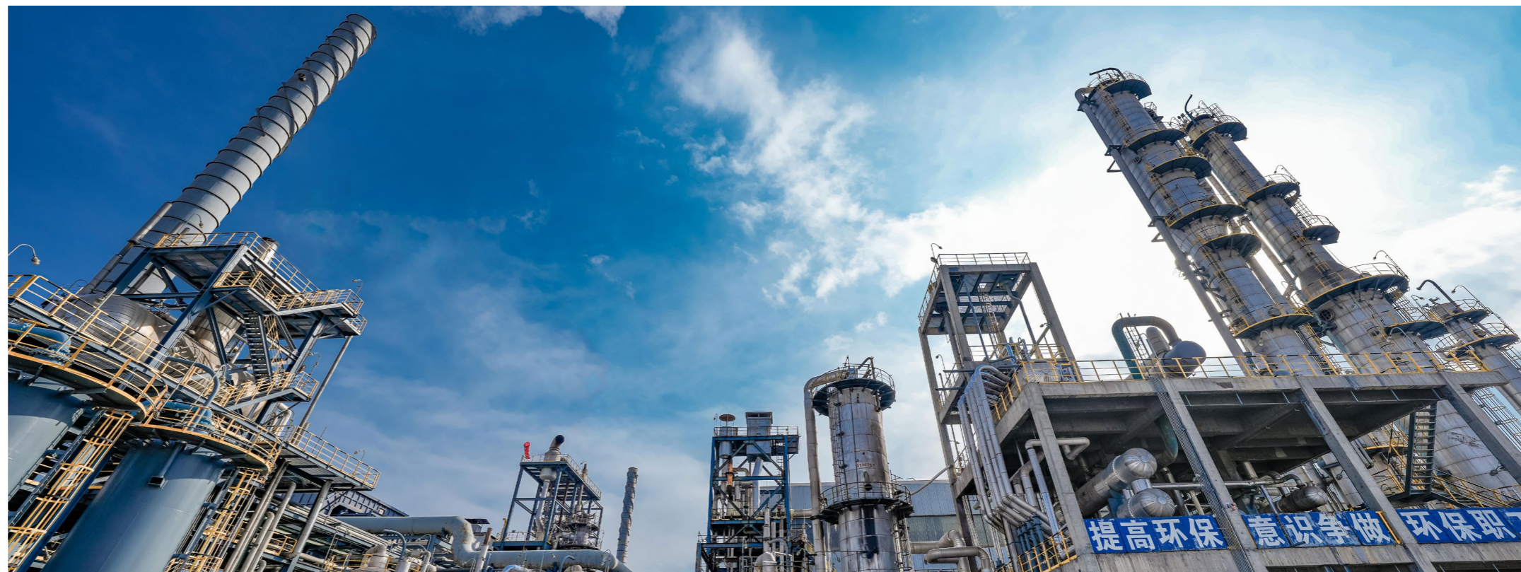
The Ammonia Synthesis Plant of Qinghai Yuntianhua Co., Ltd.
